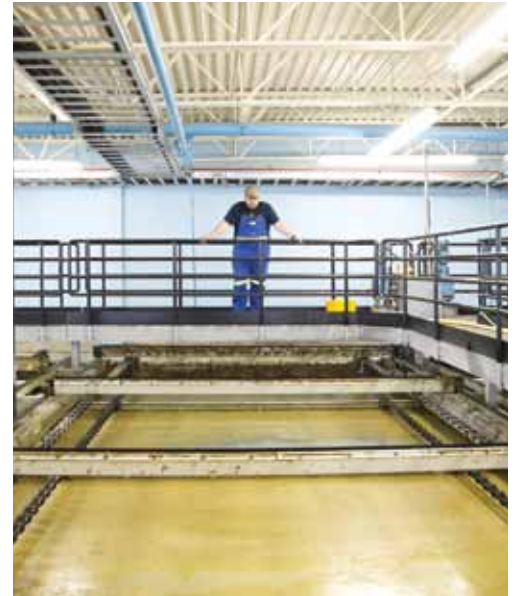
Water treatment plant dissolved air flotation (DAF) process.
