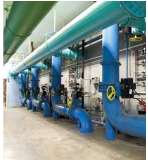
Water treatment plant filter pipe gallery.
