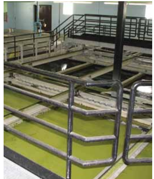
Algae removal through DAF process at the wastewater treatment plant.
