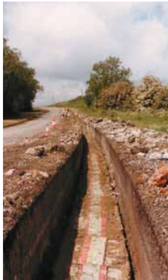
This photograph above shows an example of trenching for a direct burial transmission line in the U.K.
